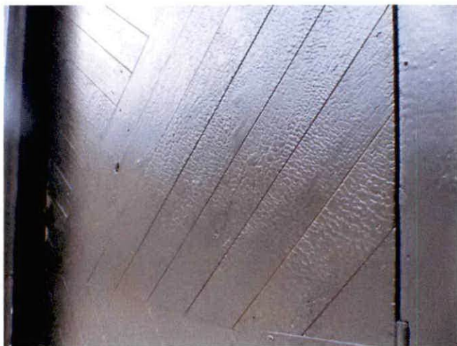
10. detail: "alligatoring" of wood planks on installed doors (6/7/2022)
