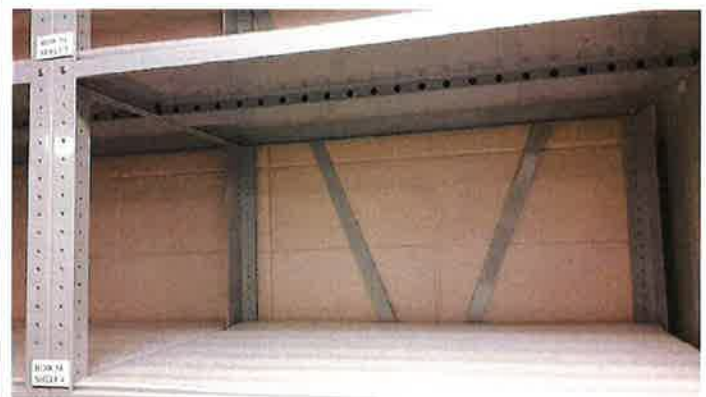
Image #20 - Underside view of mid-shelf with 36" wide brace
