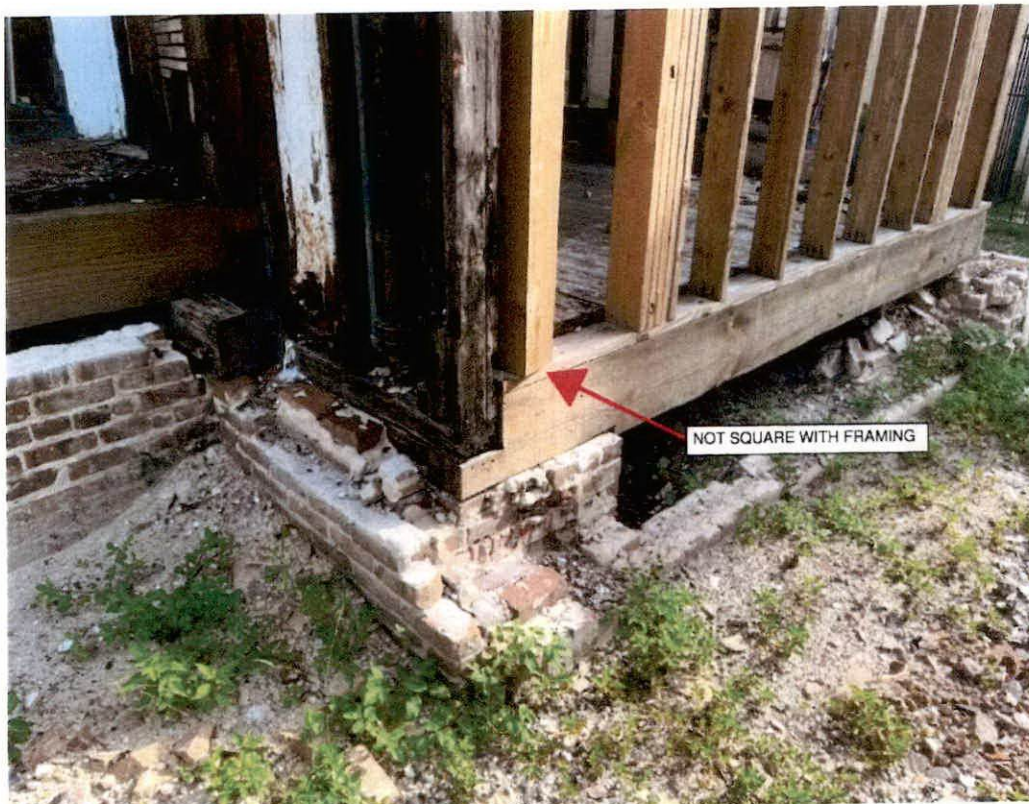
Deficiency 1. End Post (2/2)
