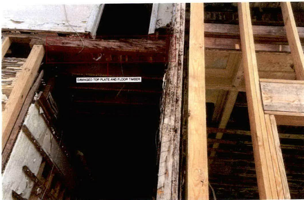
Deficiency 7. Damaged Hallway Floor Support and Top Plate
