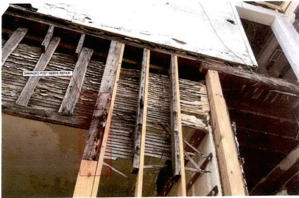
Deficiency 6. Rotted Door Post
