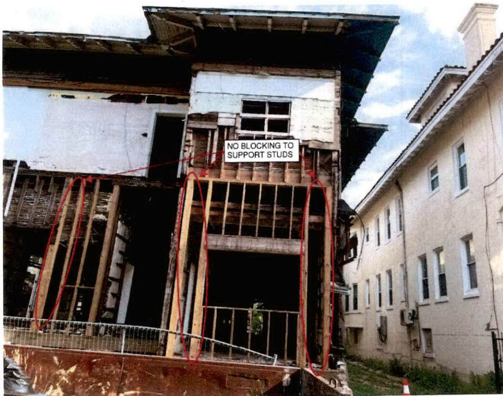
Deficiency 3. Missing Stud Blocking
