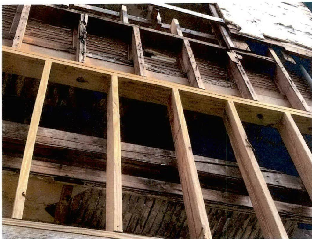
Deficiency 8. Missing Lateral Stud Connectors
