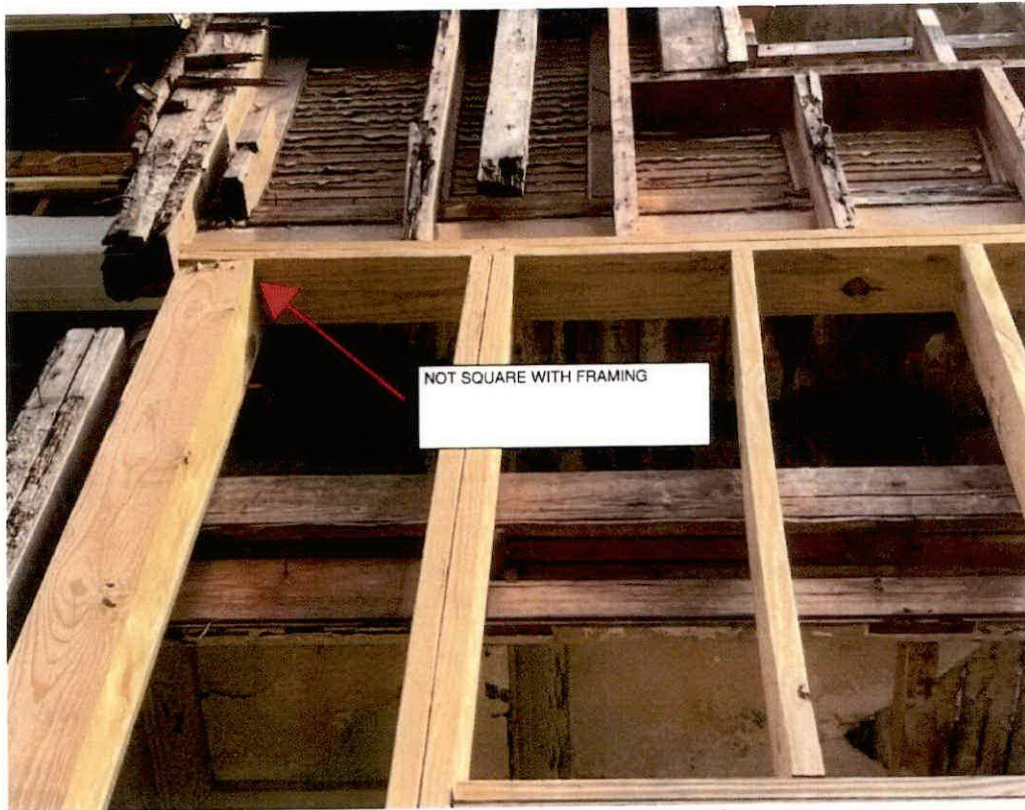
Deficiency 1. End Posts (1/2)
