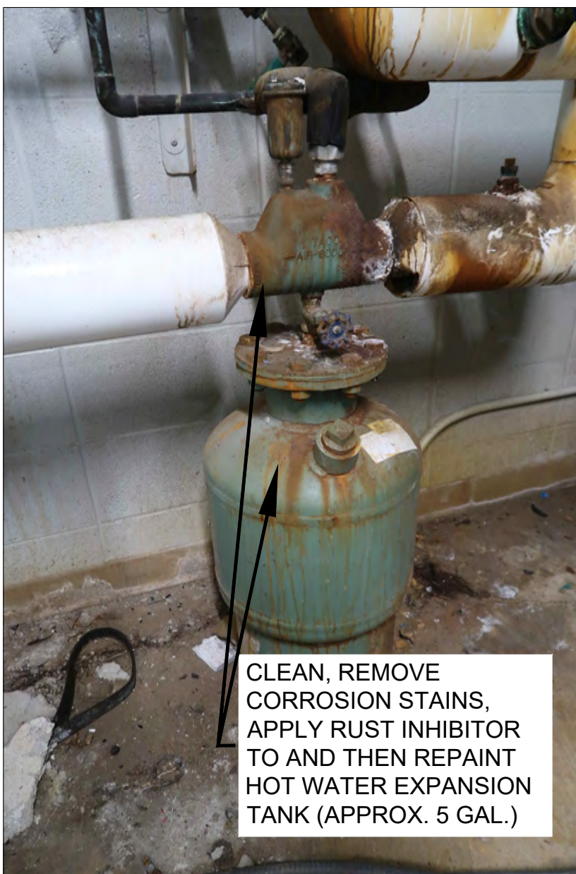
HOT WATER EXPANSION TANK NEAR AIR HANDLING UNIT AHU-1
