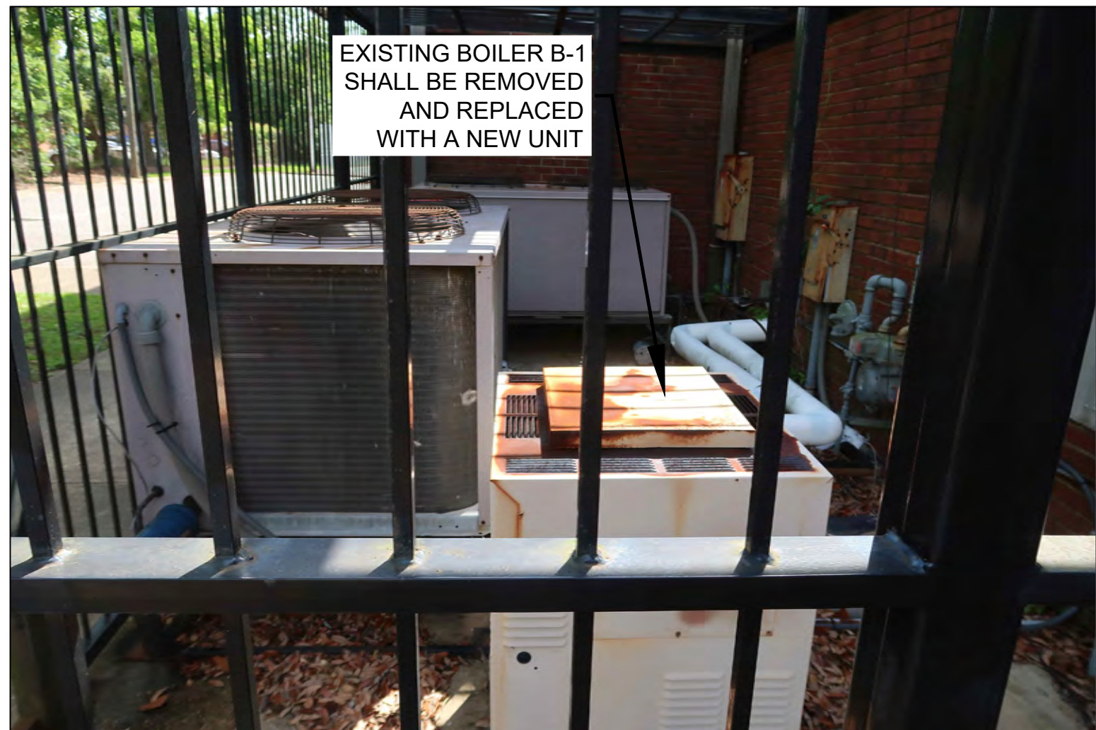
CONDENSING UNITS CU-1A, CU-1B AND BOILER HB-1
