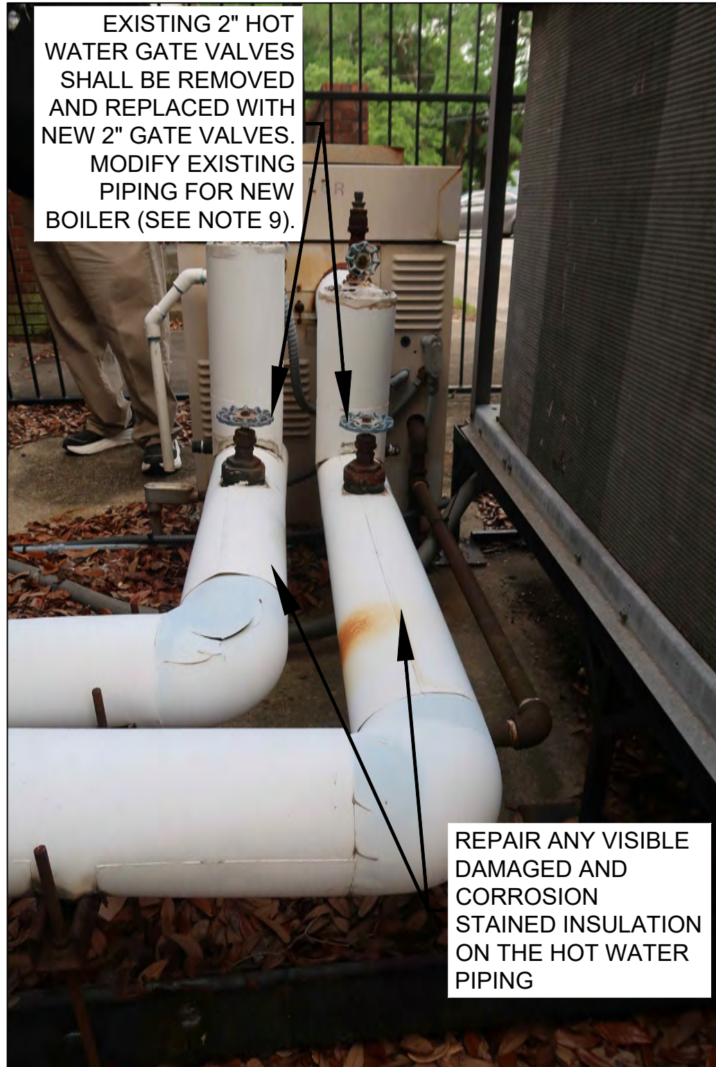
BOILER B-1 PIPING AND VALVES
