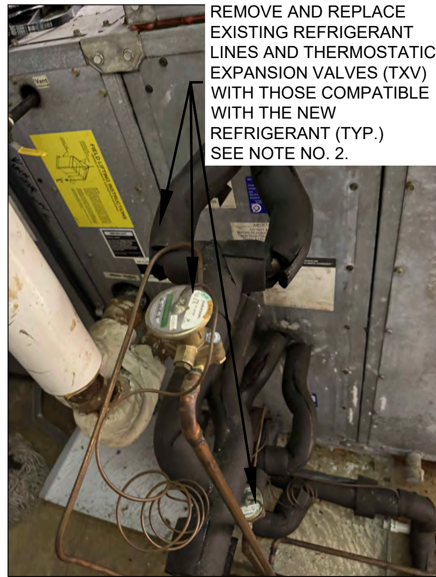
AIR HANDLING UNIT AHU-1
