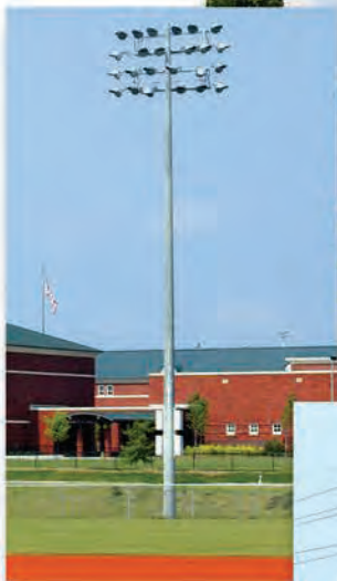
Sports, Recreational, and Athletic Facility Lighting
